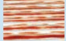
Shows significant red rust
