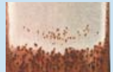
Loss of coating with the appearance of red rust on the surface near edges
